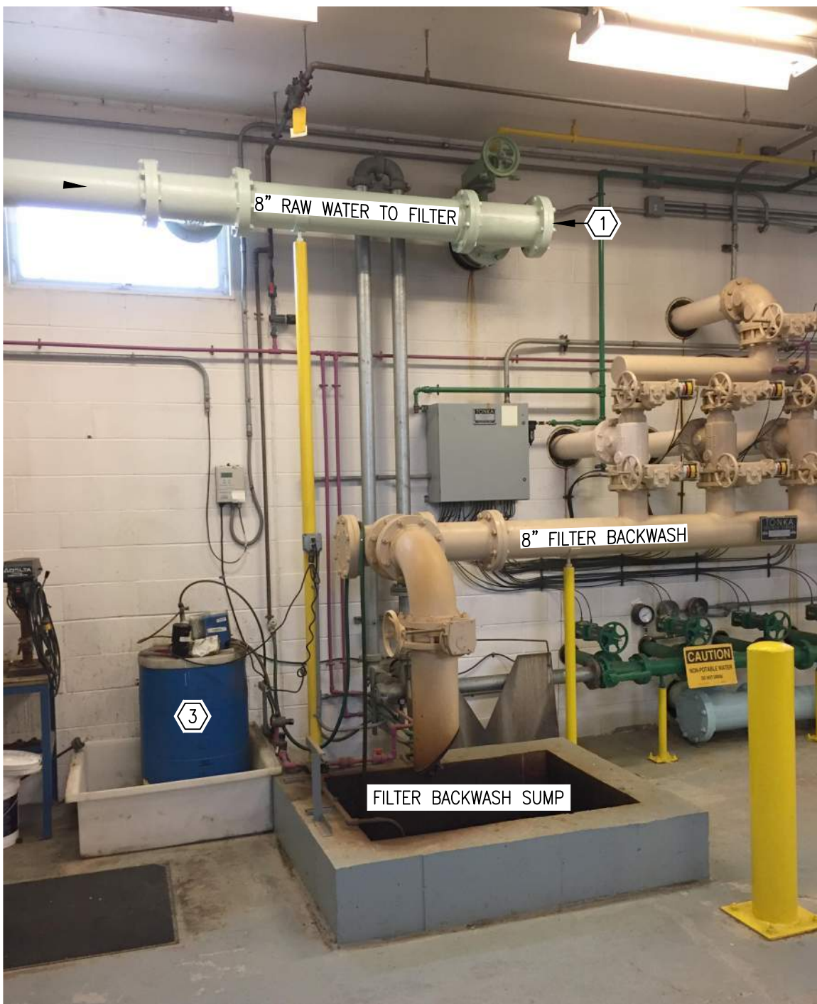
DUALATOR FILTER PIPING PHOTO NO.1 NO SCALE
